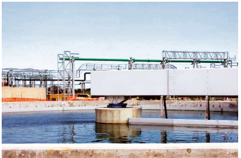
Floating scum removal with skimming troughs
