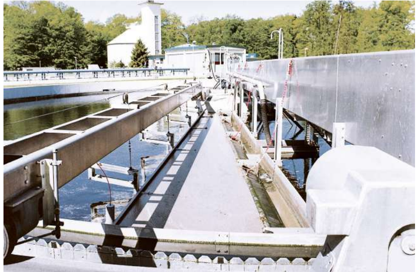
Floating scum removal with preceding submerged baffle bridge
