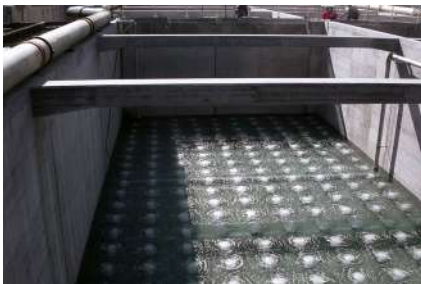
ROEFLEX® in operation
